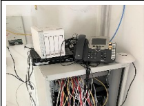
#8: Rack Cabinet and IT Equipment
