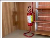
#58: Fixed Fire Extinguisher
