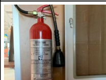
#59: Mobile Fire Extinguisher - B
