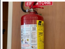
#57: Mobile Fire Extinguisher - A
