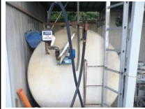
#28: Diesel Fuel Tank
