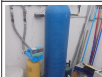
#26: Water Softener System
