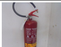
#20: N. 7 Fire Extinguishers in Powder
