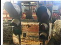
#14: traffic junctions facility
