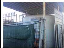
#16: Diesel distributor and Containment Basin
