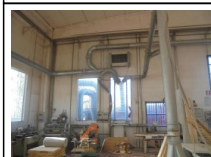
#36: Ecosplit heating system
