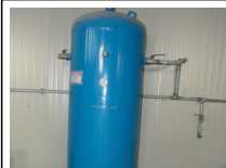
#1: Compressor, Dryer and Tank
