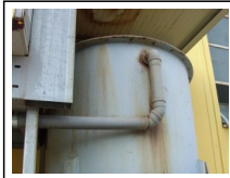
#13: Reservoir with collecting tank
