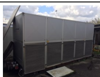
#7: Euro-Chiller External Pump
