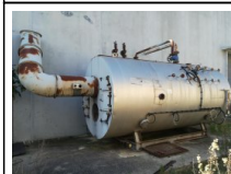
#58: Thermal Power Plant and Burner
