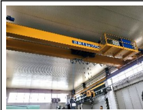
#20: OMIS 15 ton double girder overhead crane
