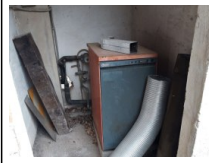
#10: Riello Atr37I Gas Boiler
