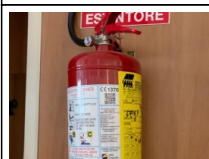
#57: Mobile Fire Extinguisher - A
