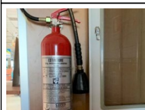
#59: Mobile Fire Extinguisher - B
