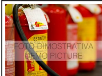
#69: N. 5 Fire Extinguishers and Hydrant
