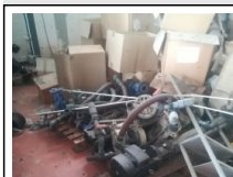
#49: Electric Motors for Purification Plant - A
