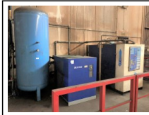
#70: Compressors, Dryers and Tanks
