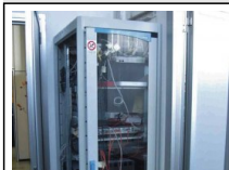
#28: IT and Electronics Equipment
