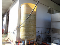
#1: N. 3 Tanks and Hydraulic Pump
